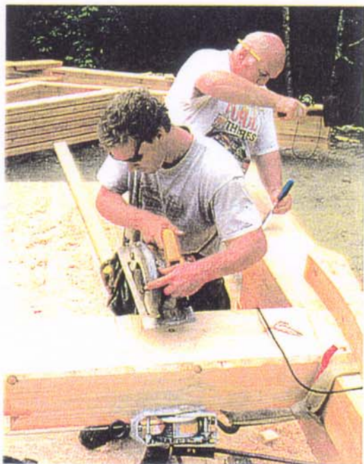
Bob North, III, and Howard Dix employ a mix of modern and traditional tools to fine-fit the joinery of a new timber frame home.
